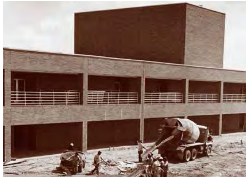
Dr. A. Rodney Allbright takes office as College President; construction begins on a new $8 million building
